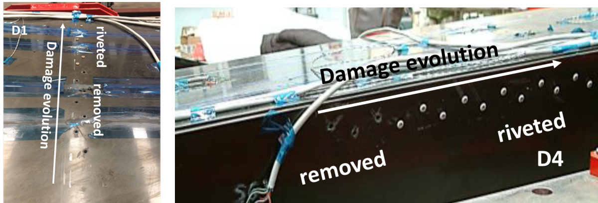
Figure 4: Detail of the removed rivets from the lower skin and the second frame(Damage D1) and between the upper skin and the lower skin (Damage D4) with the rivets partially removed
